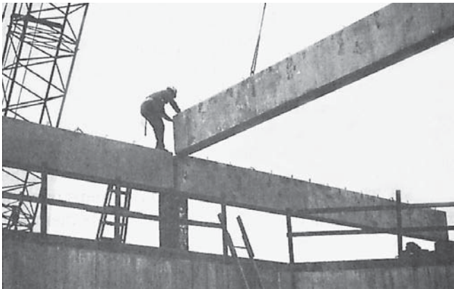
FIGURE 22.15 Precast concrete beams and panels are often formed off-site, delivered to the job site, and then set into place with a crane. © Cengage Learning 2012
