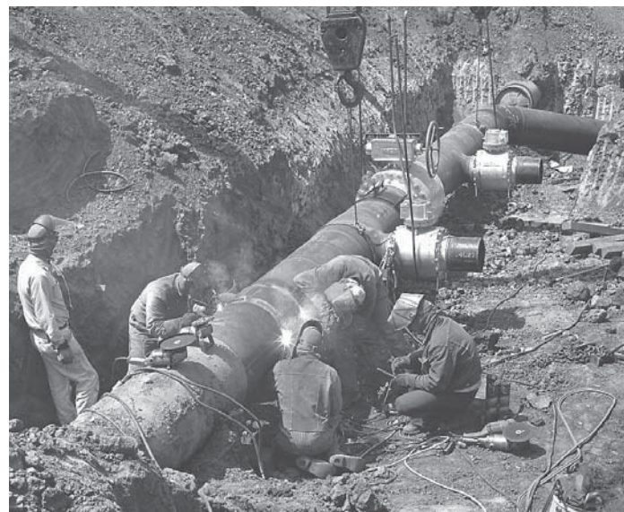
FIGURE 21.4 Underground piping supplies natural gas for homes and industries. Courtesy Pacific Gas & Electric
